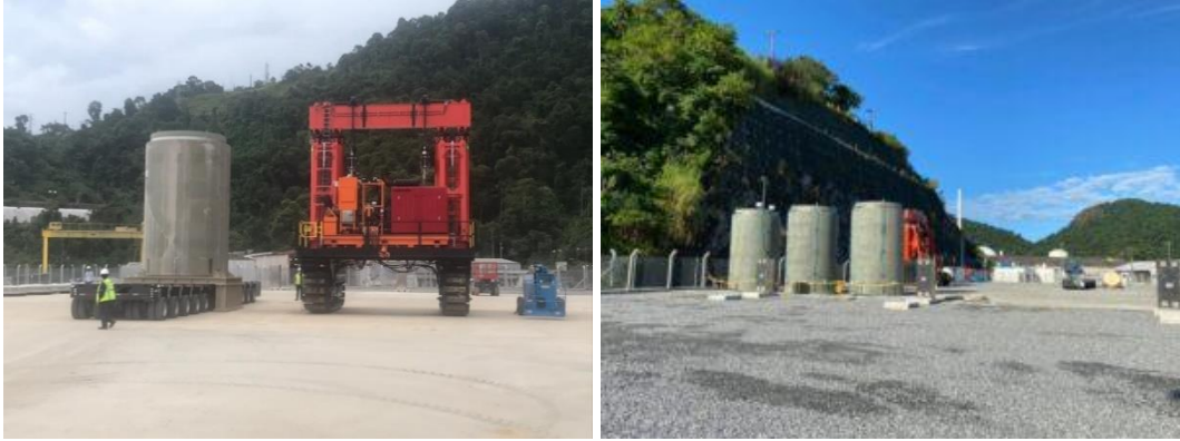
Figure 10 – Photos of the CNAAA ISFSI - Dry Storage
